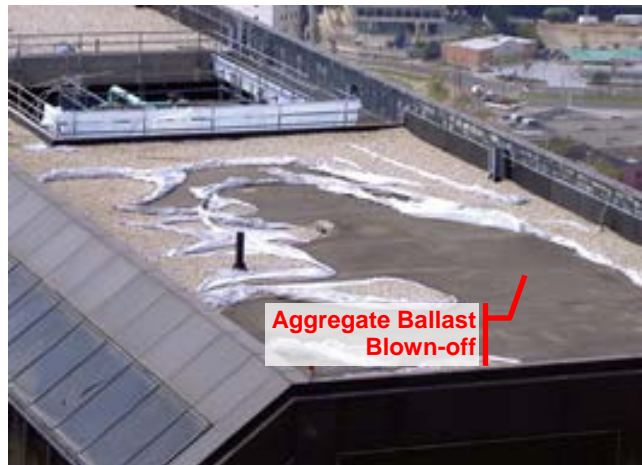
Figure 2: Aggregate ballast was scoured and blown from a large portion of the roof. (Source: FEMA 549)
