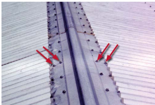
Figure 17: The ridge flashing on these corrugated metal panels had two rows of fasteners on each side of the ridge line. (Sources: FEMA "Hurricane Ike Recovery Advisories")
