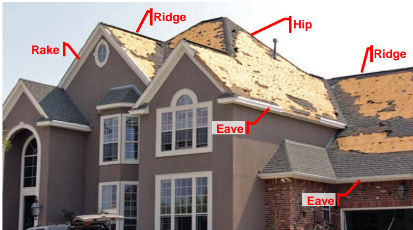
Figure 10: Asphalt shingle roof blown-off. (Source: FEMA P-55 / Volume II, "Coastal Construction Manual")
