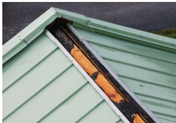
Figure 18: The ridge flashing fasteners were placed too far apart. A significant amount of water leakage can occur when ridge flashings are blown away. (Sources: FEMA "Hurricane Ike Recovery Advisories")
