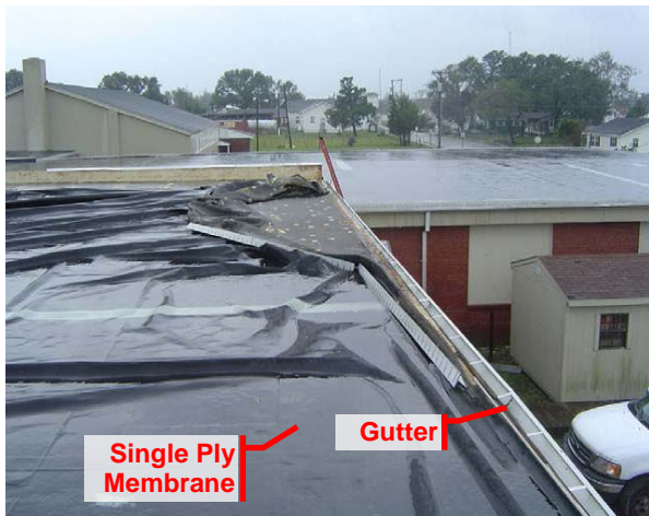
Figure 5: Single Ply Membrane (SPM) peeling due to gutter failure.
