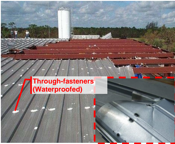
Figure 11: Failure of through-fastened metal panel systems due fasteners excessive fastener spacing at perimeter and corners. Metal panel torn off over the fastener head.
