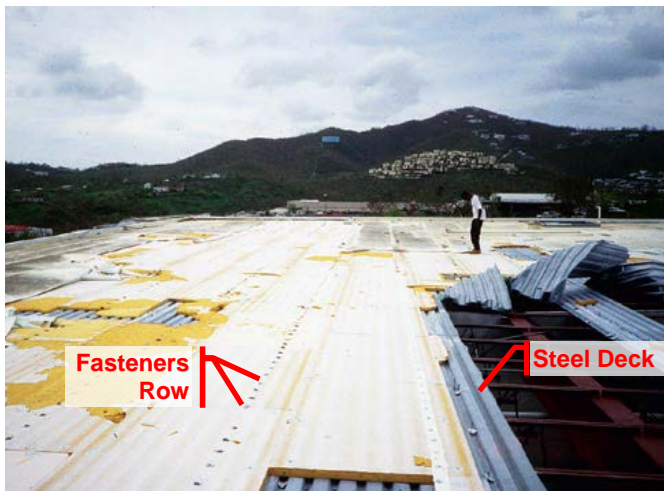
Figure 7: Fastener rows of the mechanically attached single-ply membrane ran parallel to the top flange of the steel deck. The deck fasteners were overstressed and a portion of the deck blew off and the membrane progressively tore. (FEMA 543)
